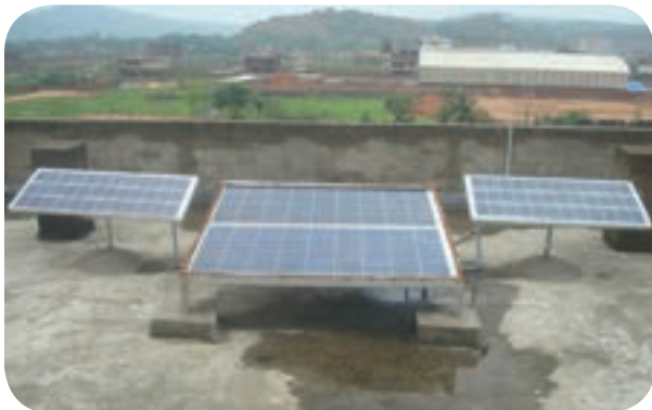
Solar System (150W) installation at Lokhra
